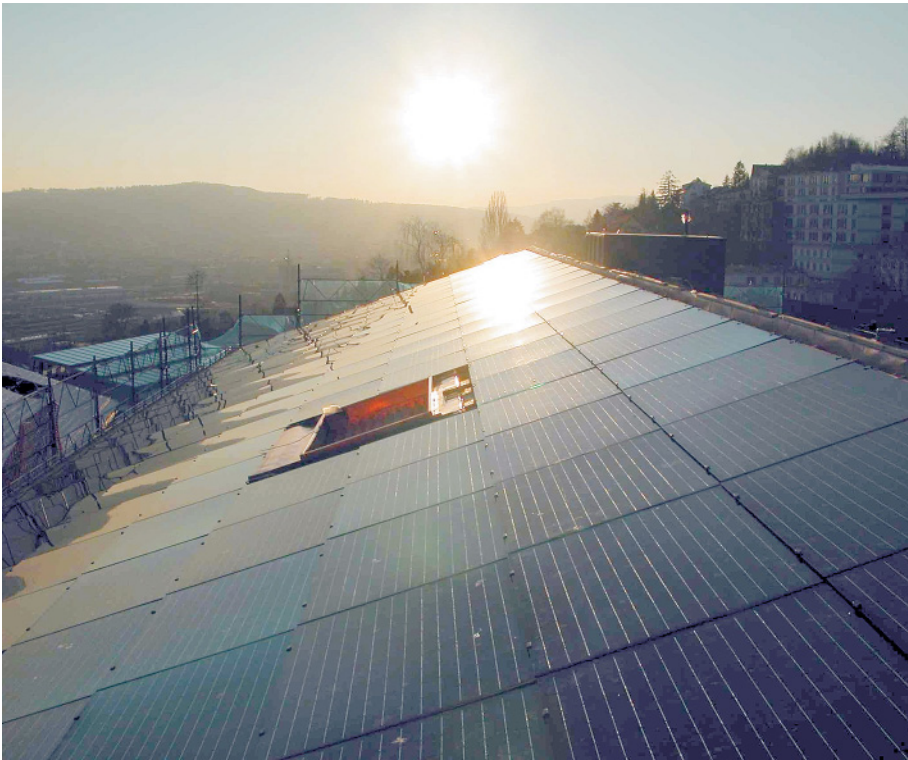
Anlage Application Application Waidspital, Zürich (CH)
